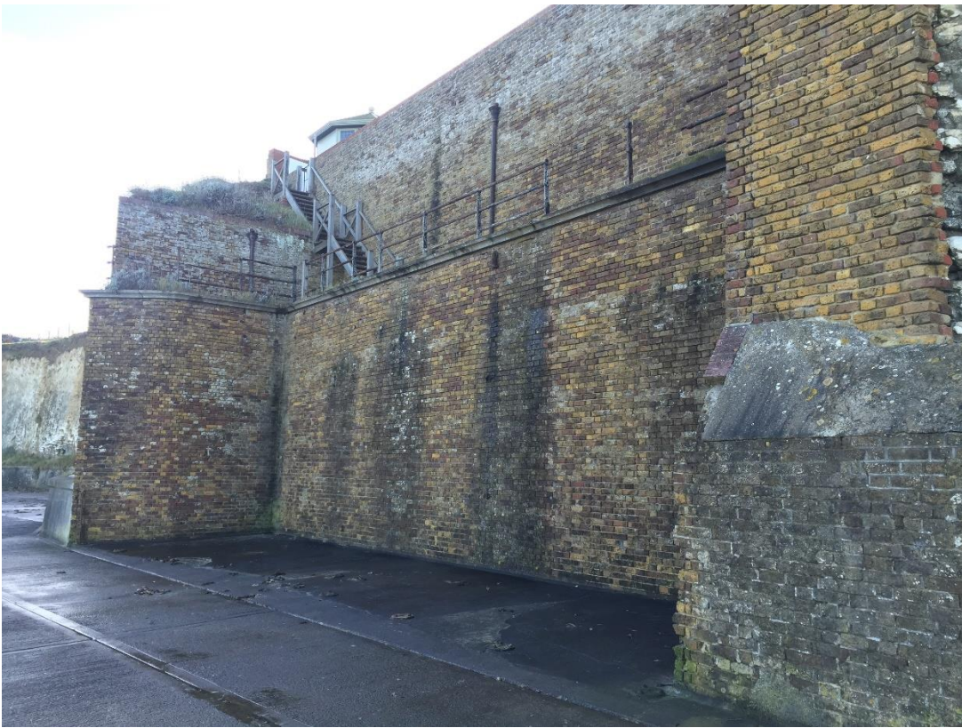
Private stairs at one point? Stairs from garden to deck still there, but railings rotting so doubt it's used. Would the brickwork be part of the cliff repairs we have archived? (1913 maybe).
